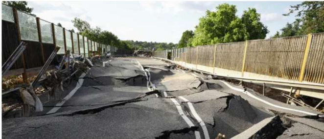
Damaged road in Germany after flooding in 2021. 1
